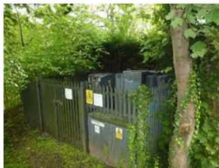
Substation No. This number will appear on the white sign, usually on the door or gate.
